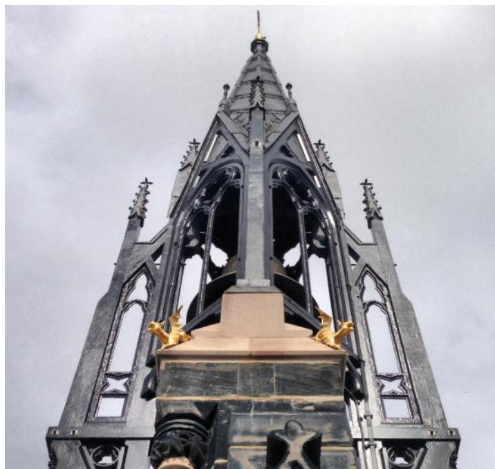
Above: Restoration works to the spire St Vincent de Paul, Liverpool (Grade II* listed).
